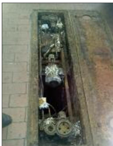
existing, worn out lift
